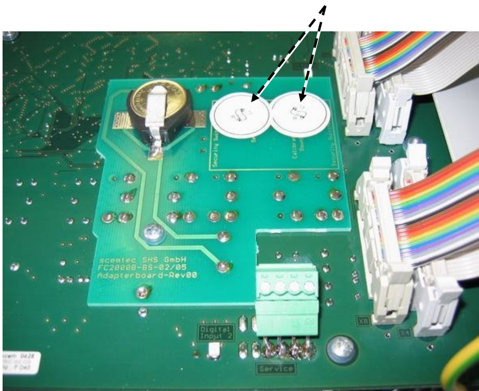
Typical Sealing of Calibration Switches
