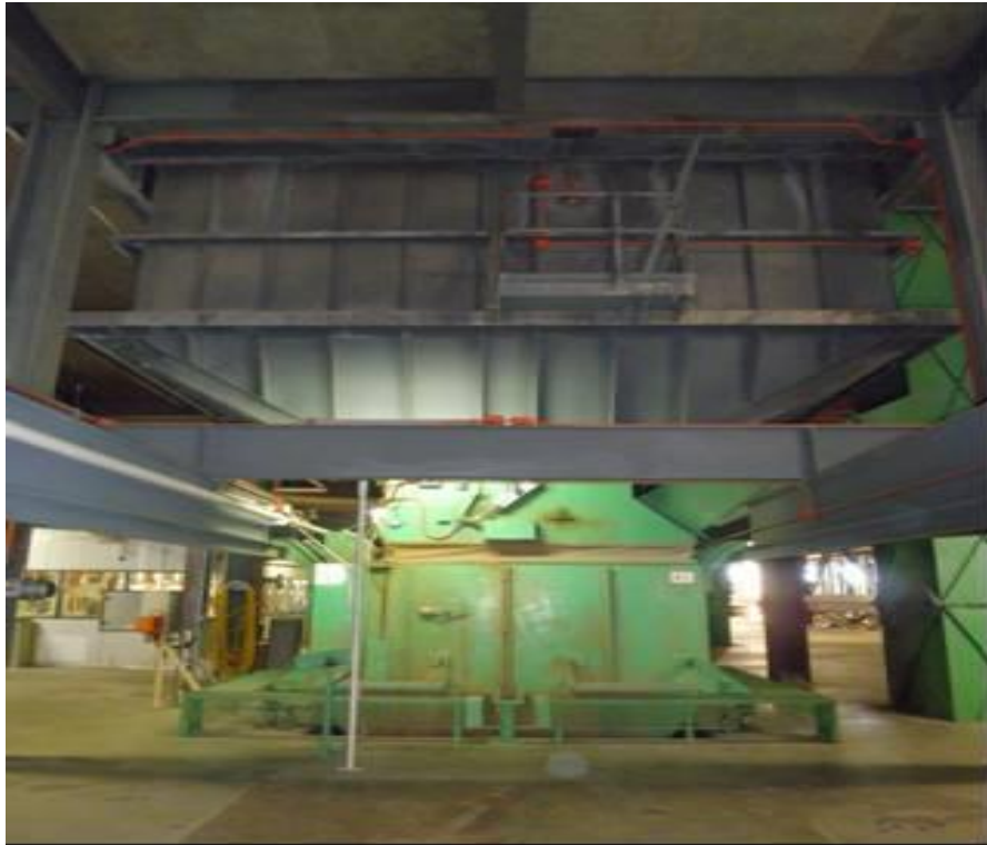
CBH DTAW1 Totalising Weigh Hopper/Weigh-bin (Kwinana)
