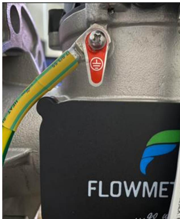
Grounding cable attached to meter grounding tear
