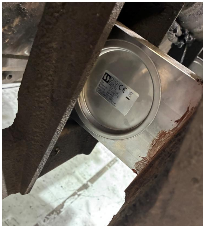
Load Cell (Installed Behind the Load Receiver Frame)
