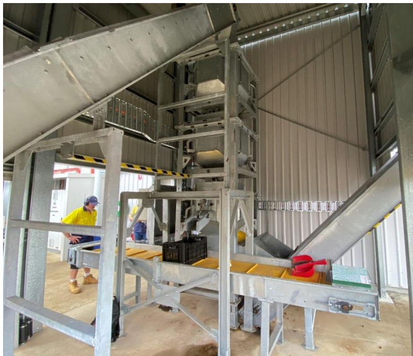
Typical Integration Installation With Sampling Crate Conveyor
