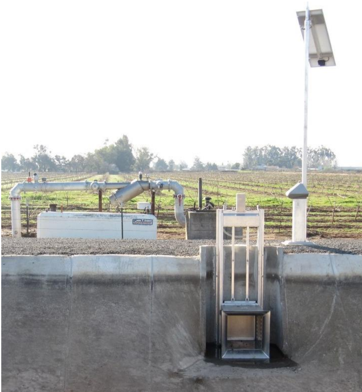
Example of Rubicon SlipMeter installed into a headwall
