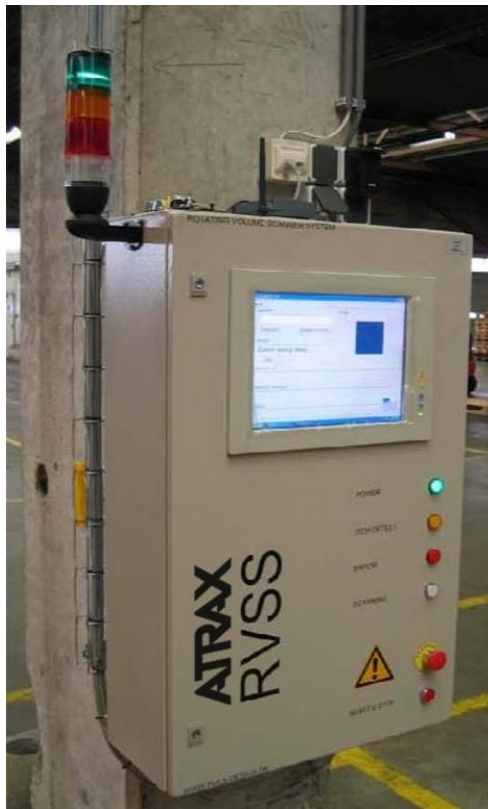
(a) RVSC Control Unit With an SIPC Touchscreen
