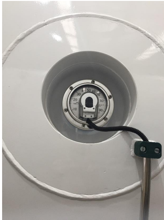
Rochester Remote Ready Dial, R3D level indicator
