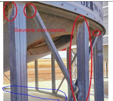
Picture 5. This picture is a close up of rusted Duragal® 15 year silo stand.
