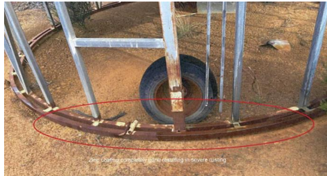
Picture 7. This picture is a close up of rusted Duragal® silo stand.
