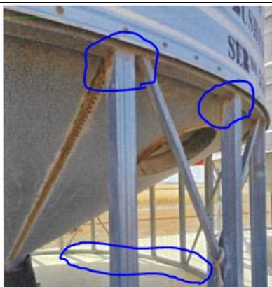
Picture 4. This picture shows a relatively new silo around 15 years old made from ALLGAL® with significant corrosion of the silo legs.
