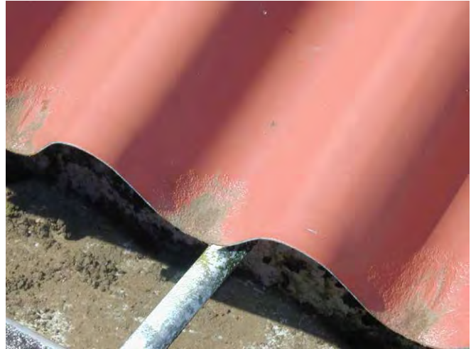
Silt accumulation on a panel without a drip edge. Blistering of the paint is an early sign of corrosion.
