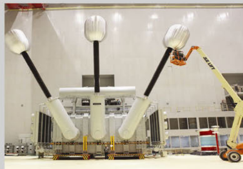
宝鸡电厂 SFP-780MVA/800kV ASA Baoji Power Plant SFP-780MVA/800kV ASA
