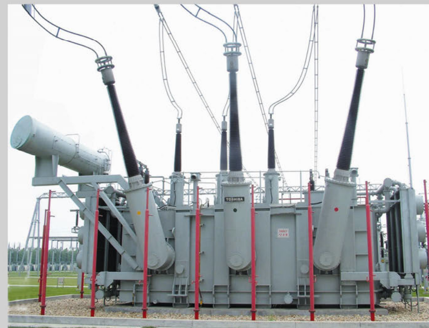
江北变电站 OSFPS-750MVA/500kV Jiangbei substation OSFPS-750MVA/500kV
