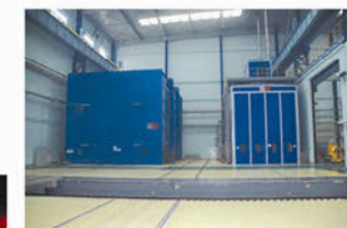
喷丸室和干燥室 Wheel abrator cabinet and drying room
