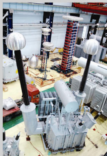
研发变 Research and development transformer
