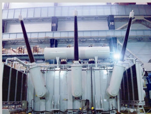
铜陵电厂 SFP-1140MVA/500kV Tongling Power Plant SFP-1140MVA/500kV
