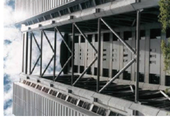
Steel pipe brace
